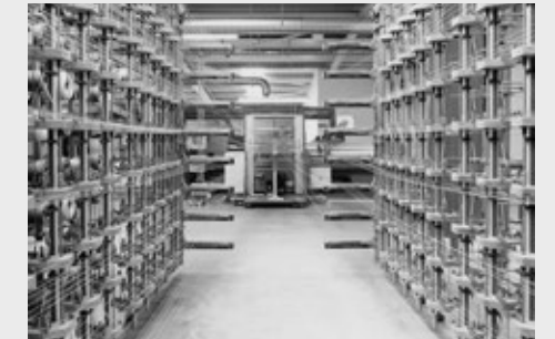
027 Kvadrat warehouse in Ebletoft, Denmark 028 Google's data center infrastructure
