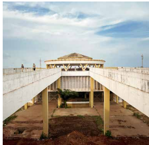
009_ARLL_109 Round pavilion and access ramp in disrepair, March 2023
