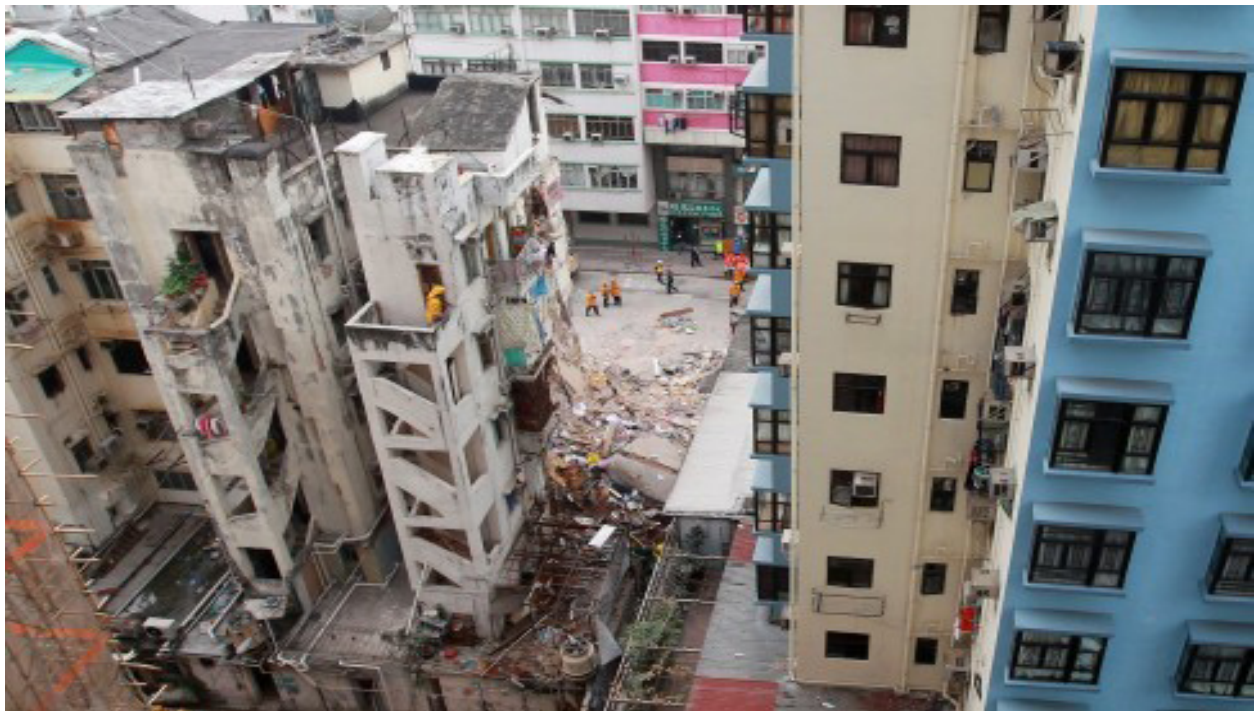
Figure 2.3 Deteriorating Conditions in the To Kwa Wan (Wan 2014)
