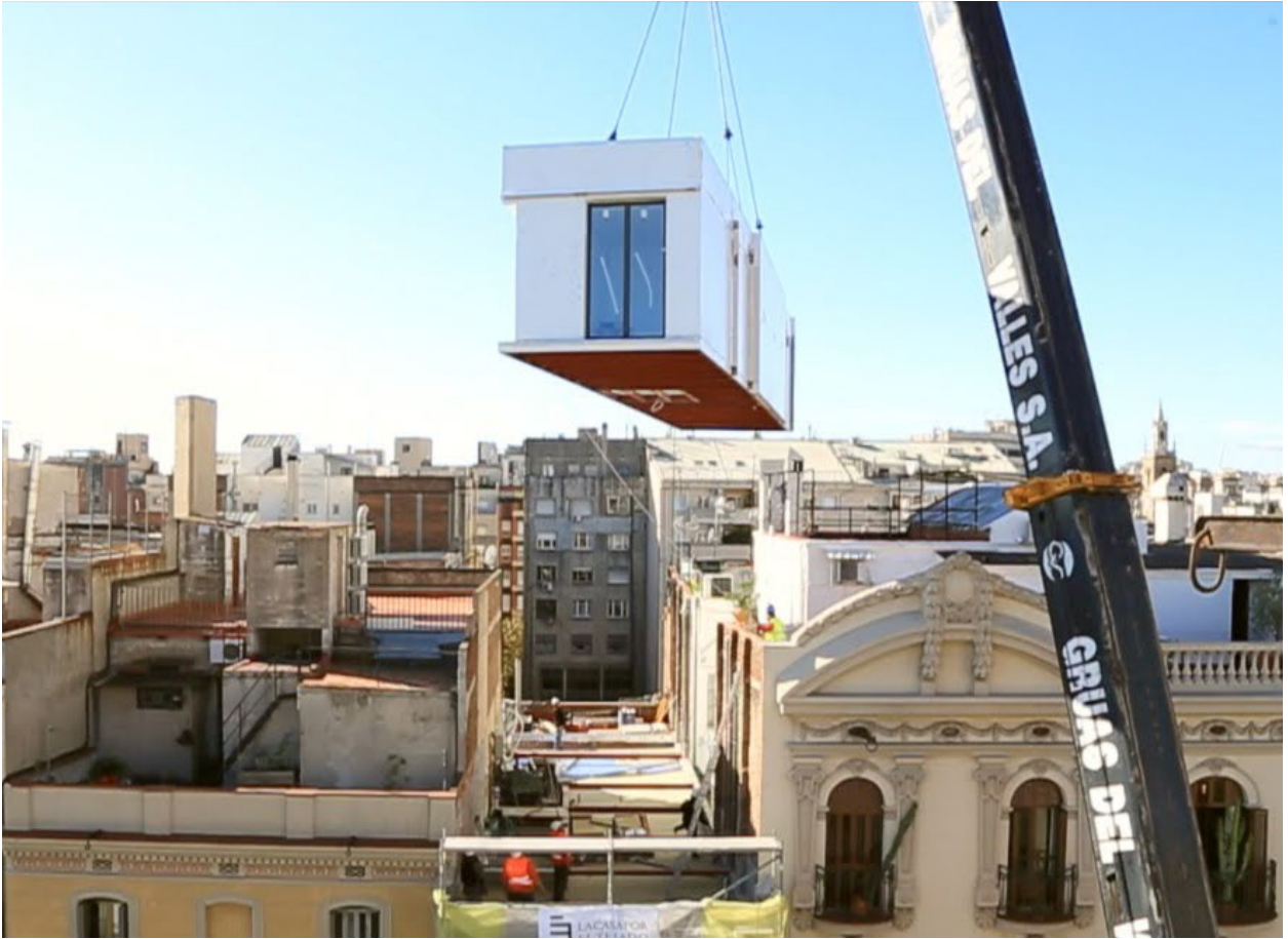
Image 06 | La Casa por el Tejado, rooftop ADU project in Barcelona. Modular rooftop unit being lifted into place by crane.
