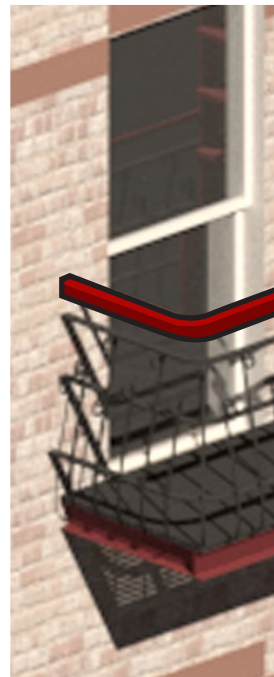
2C EXTEND RAILING HEIGHT TO CURRENT SAFETY STANDARDS.
