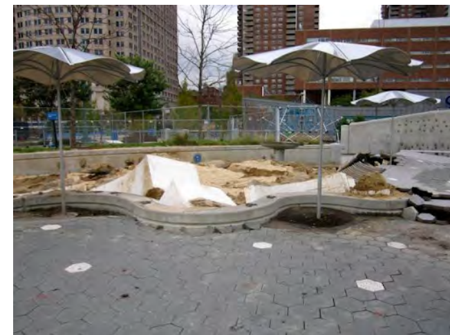
Superstorm Sandy Damage Hudson River Park
