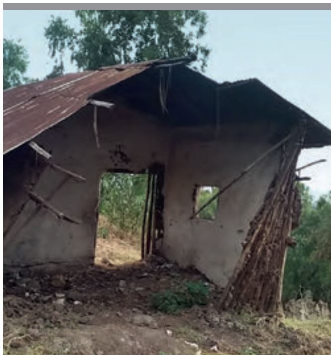
A typical gojo in “poor” condition
