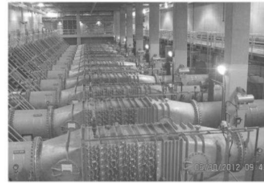
and passes through a 1.5 billion dollar treatment facility
