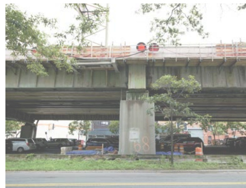
Poorly Maintained Roadways
