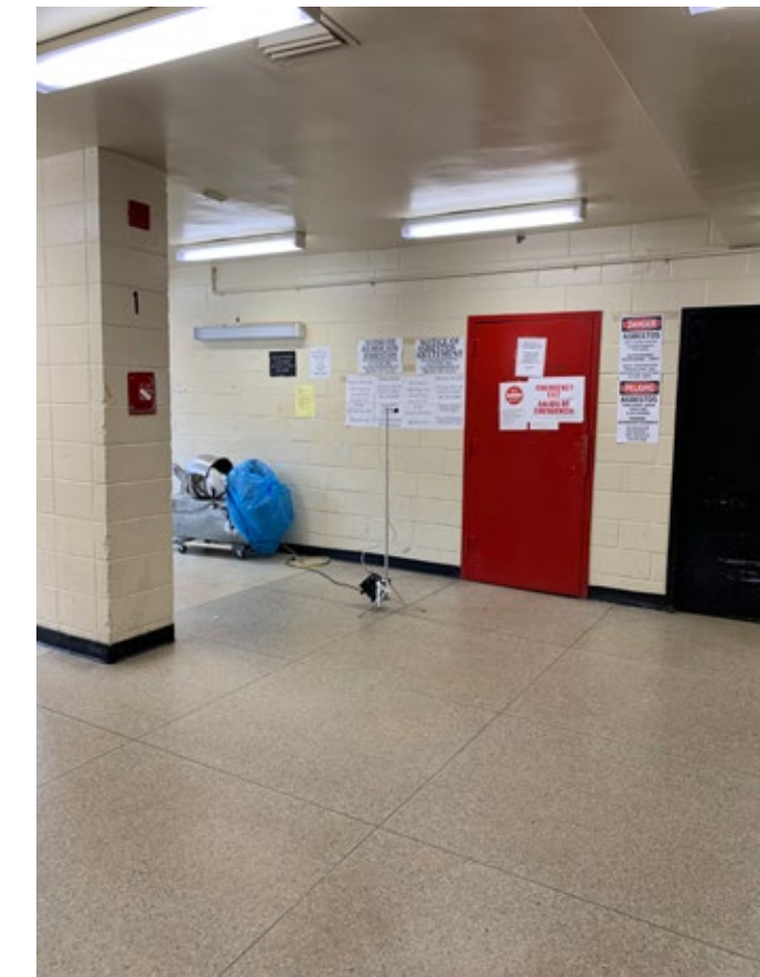
Figure D & E: Equipment and signs for asbestos abatement at Courtlandt Houses building 1. Photographs by the author.
