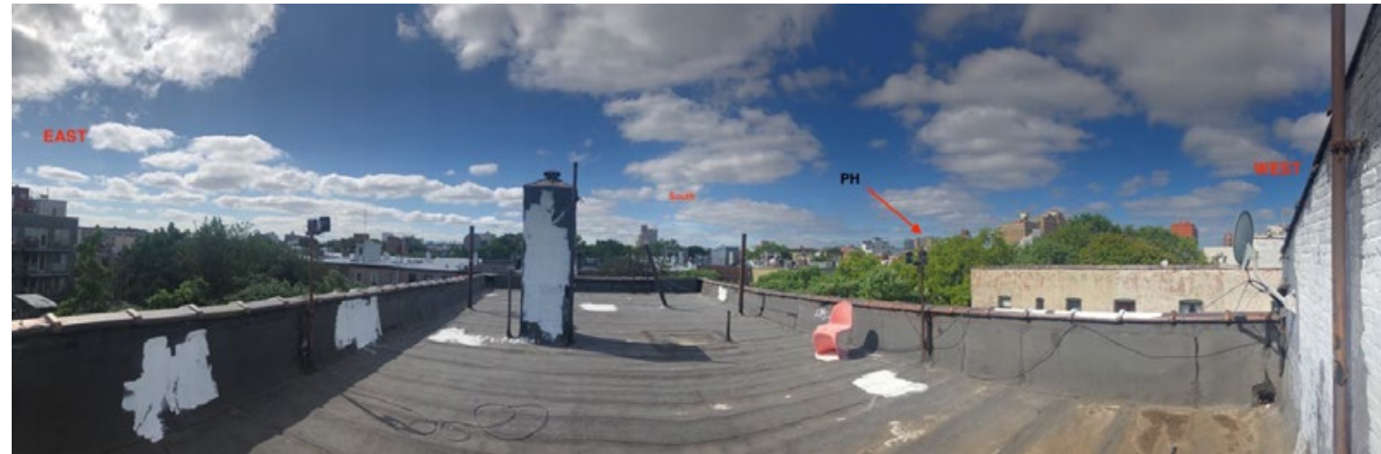
Figure A: The roof of my old apartment building as pictured by a volunteer NYC Mesh technician. Photo courtesy of NYC Mesh.
